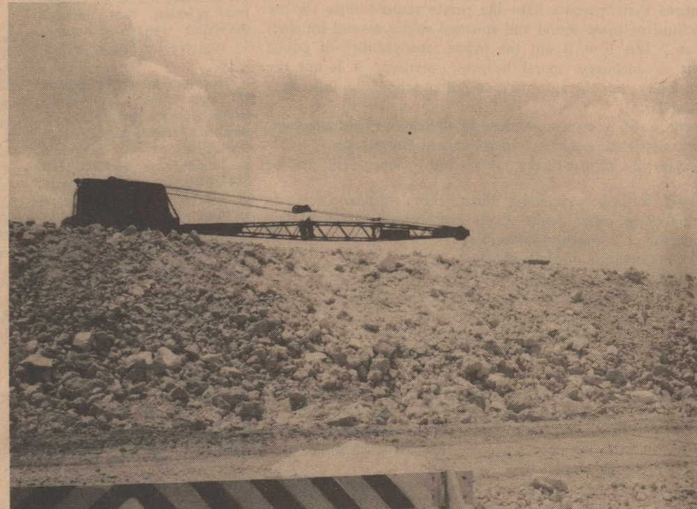
ROAD CONSTRUCTION SOUTH OF TOWN causes blackout just after noon Monday. During operation, this large crane managed to pull down several electrical lines, shutting off electricity to much of the town including downtown businesses. However, utility service men had the electricity back on shortly, and took care of the hot lines across the tip of the crane and the roadbed.
