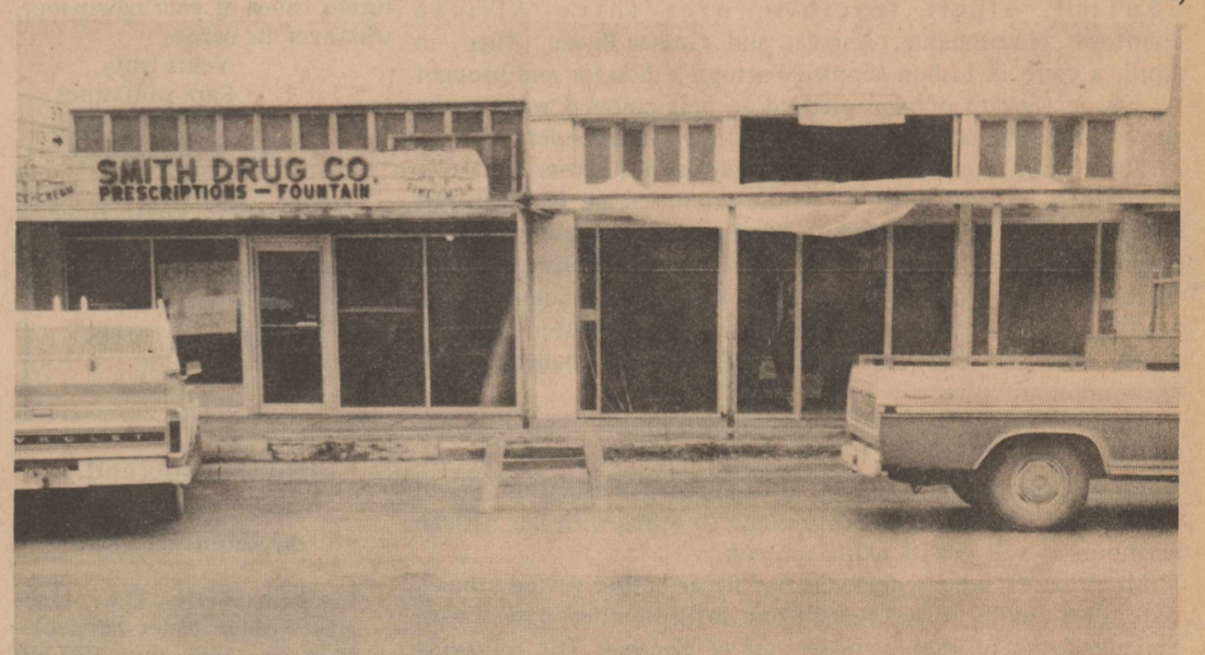
END OF AN ERA -- The Smith Drug building and the building which housed Parker's Cleaners for half a century are being remodeled. Already the clock which was a landmark atop the awning of the cleaning shop is gone. The Smith Drug sign and the awnings will come down this week. New glass fronts have already been installed. A men's wear store will soon open in the drug building and a savings and loan branch in the other.
