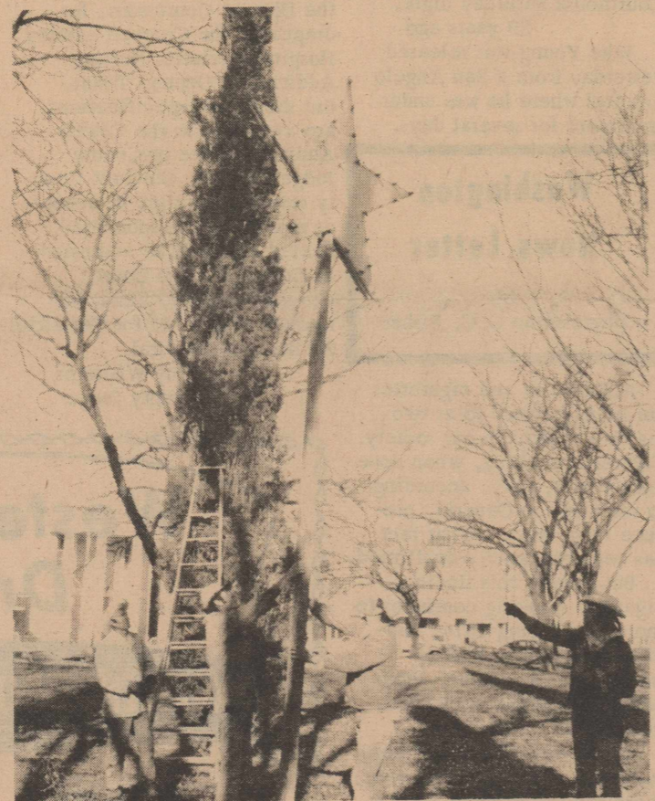
CHRISTMAS DECORATIONS were completed in the downtown park Tuesday with installation of the large lighted star which can be seen from most parts of the town. Water District employees complete the job and it takes four men to get the heavy star in place.
