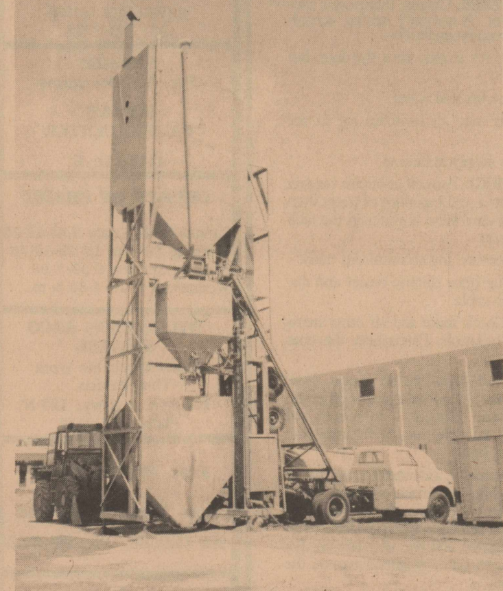
GIANT MIX-MASTER -- This huge cement mixer will be used for the tons of concrete which will go into the building of the in-town section of IS 10. The one piece of equipment dwarfs the trucks surrounding it and stands several stories above the Ozona Wool and Mohair Co. building where it is standing.
