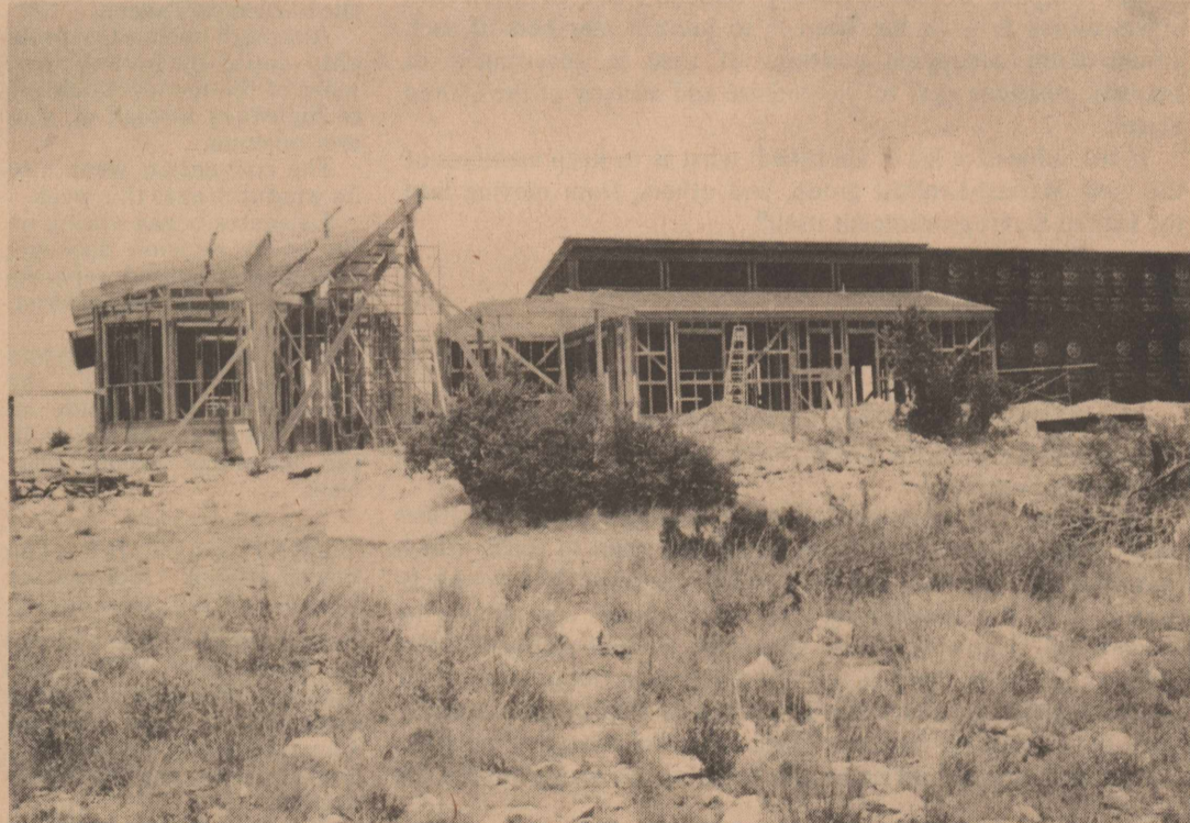
HOTEL? MOTEL? RESORT CENTER? Neither. This sprawling piece of construction is the future home of Mr. and Mrs. Bob Childress. It is under construction atop the West hill in Ozona across from the Tom Mitchell home. Just one of several new homes under construction in Ozona, but by far the most interesting for the construction observers.
