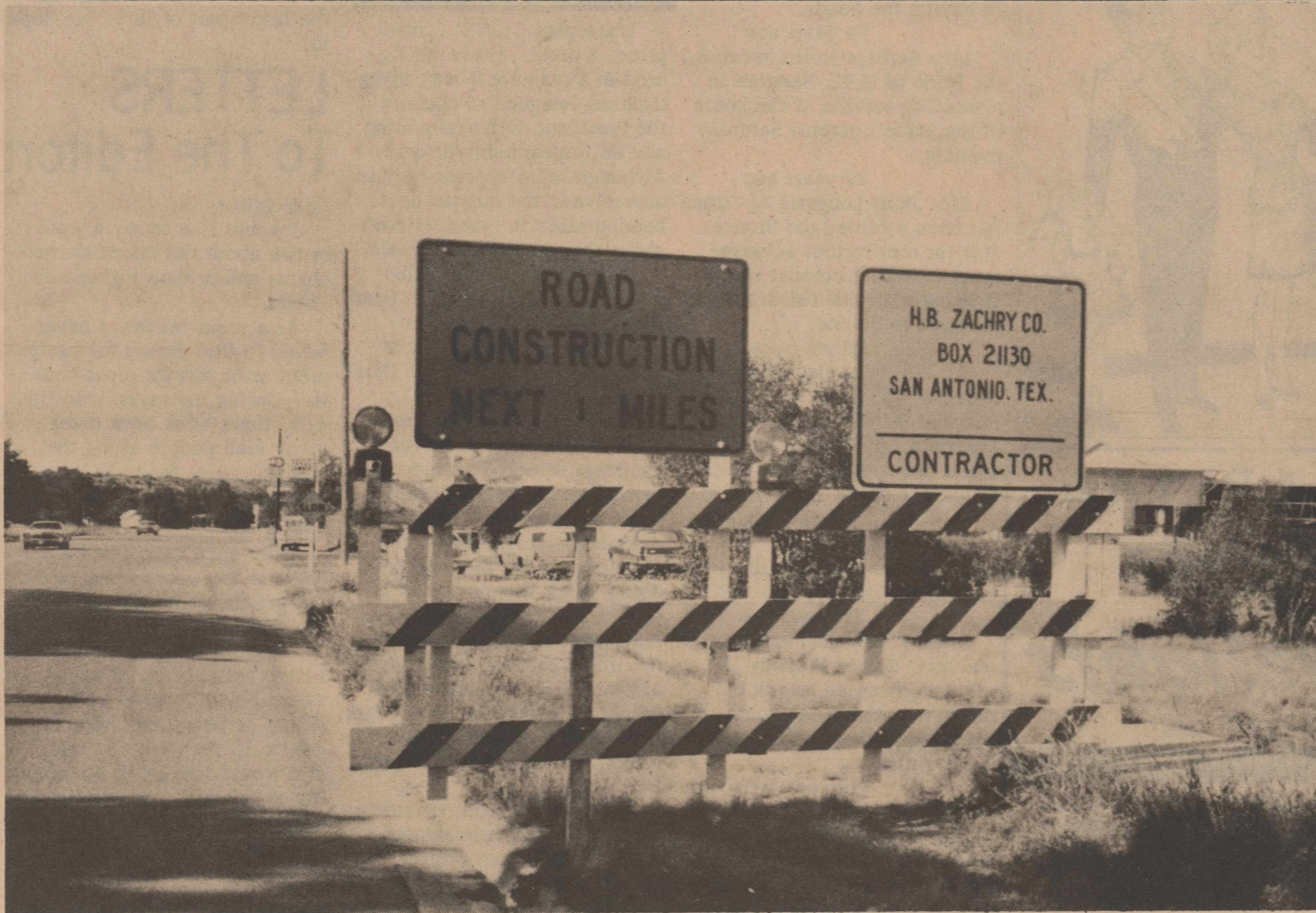
SIGNS WENT UP BEFORE THE WEEKEND AT SITE OF IS 10 construction in the south part of Ozona. The projected finish date is 19 months. The highway through this part of Ozona will be elevated to a height of 20 feet and State Highway 163 will
