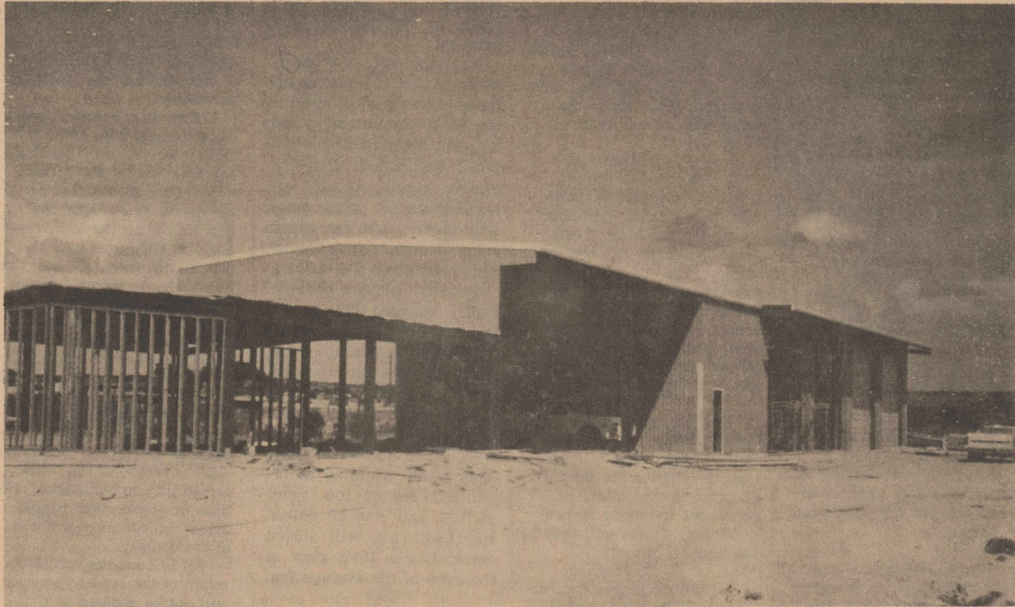
NEW QUARTERS FOR COUNTY MAINTENANCE DEPT. will soon be ready for occupancy. The new steel and brick building is a far cry from the old "county barn" which still stands in the path of IH 10 through Ozona and is still being used by the county
