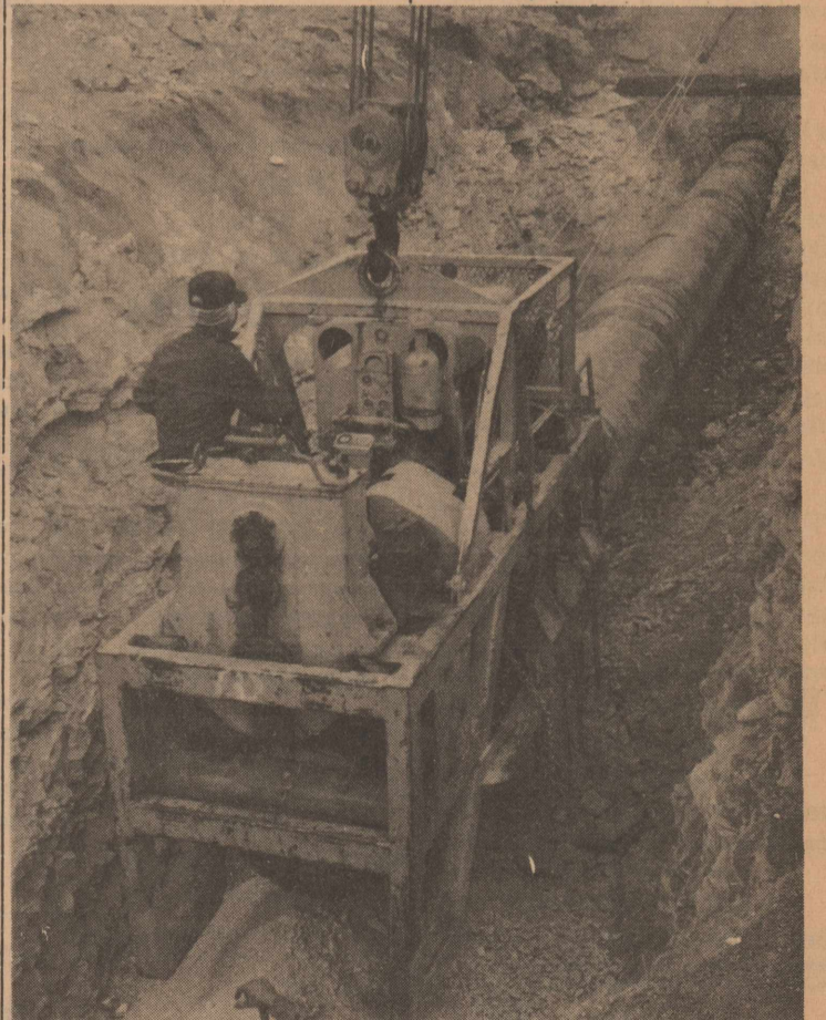
BIG MACHINES DO BIG WORK. AND this is one whale of a machine doing a tremendous job four miles south of Ozona last week. The machine pictured is driving a bit which is boring a hole through solid rock under State Highway 163 to carry the 36-inch pipeline being laid across this county by McVean and Barlow, contractors. The pipeline is part of the line being laid from New Braunfels to the Coconosa area north of Fort Stockton in Pecos County. The pipe following the auger is 42 inches in diameter and will remain under the road as a carrier for the 36-inch pipe. The machine augers the cuttings out of the hole (note cuttings beneath operator) and drives the pipe ahead as the hole is cut. The boring machine, held up by a winch line from a bulldozer parked on the side of the big ditch, drives the auger by gear wheels. The big driving gear may be seen beneath the machine. It took more than two days to drill the 100-foot plus tunnel under the highway.
