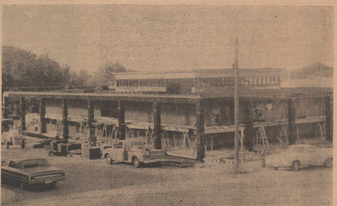
BUILDING PROGRESSES — The new home of the Ozona National Bank is slowly taking shape as building contractors reach the stage of tedious finishing operations. The black polished granite columns and trim are complete and workmen are shown on scaffolding preparing to plaster the ceiling of the porch.
