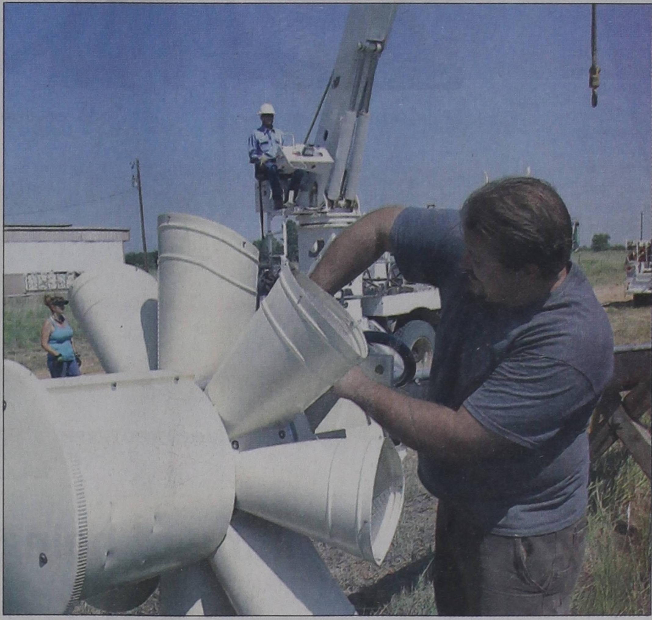
Dan Shaney of Storm Sirens, Inc., prepares part of Howardwick's new storm warning system for installation Tuesday morning.
