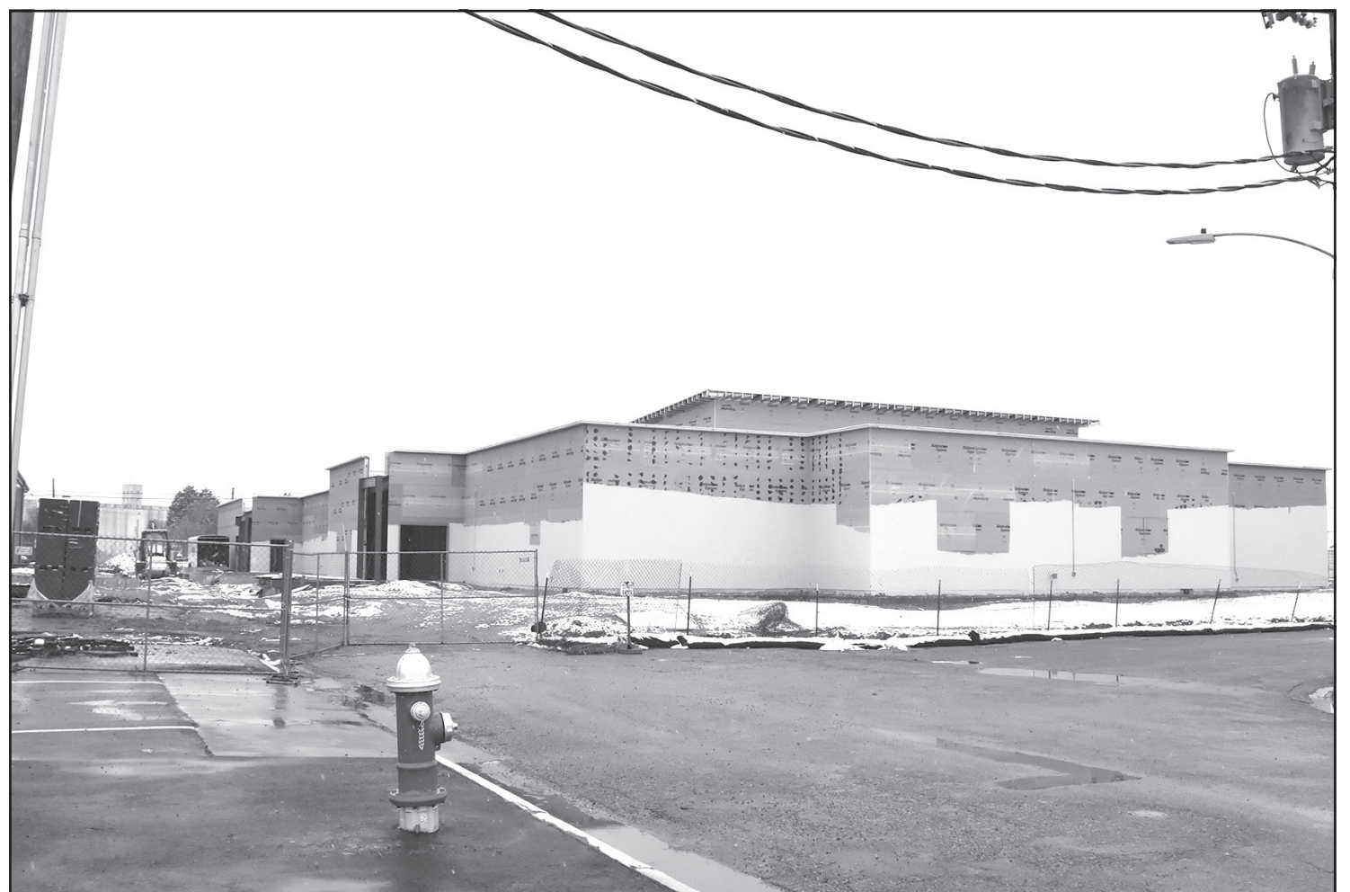
The new Primary School building is beginning to take shape. Construction is pretty well on schedule considering the COVID-19 pandemic. Estimated completion date is July 2021.
