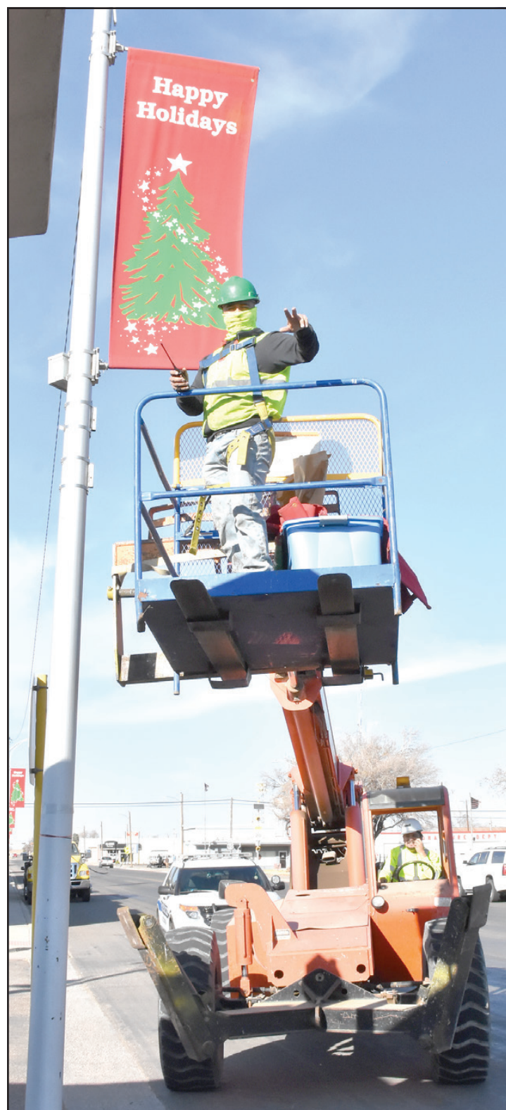
Trevino Welding & Millwright employees Raul Licerio (above) and Pedro Gomez (below) are shown installing banners and lighting on Main Street last week. TW&M LLC donated the manpower, time, and equipment for the annual holiday installation.
