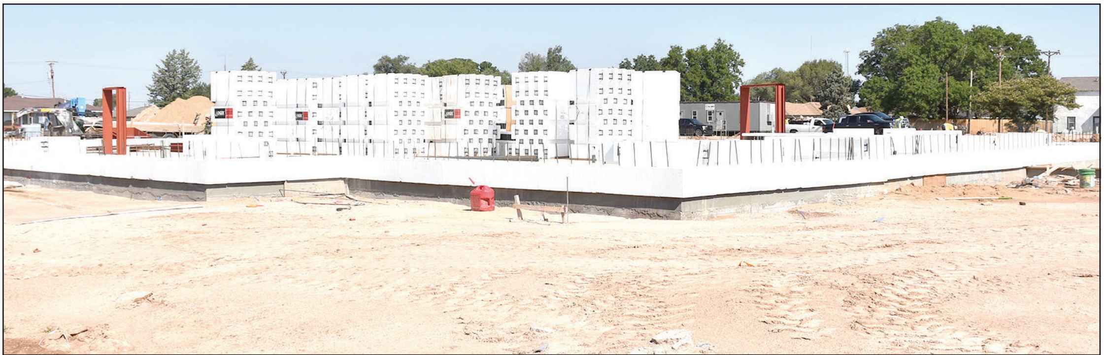
The concrete pad was poured last week for the storm shelter portion of the the new Primary School building. The next step is framing and sheathing which will begin soon.
