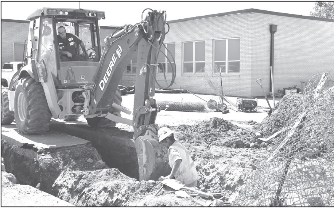
New Primary School Campus: Crew members worked on concrete footings, grade beams, MEP rough-in, and slabs. Work is slightly behind schedule but the scheduled completion date for the new Primary School is not until July of 2021.
