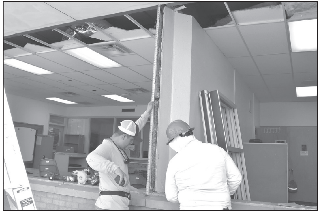
High School Campus: Workers replaced windows at the High School. The building will also get corridor ceiling, bathroom, and waiting & entrance area remodels. Work is scheduled to be completed by the middle of August. Work on the new band hall/storm shelter is also slightly behind schedule. Completion is set for the end of December of this year.
