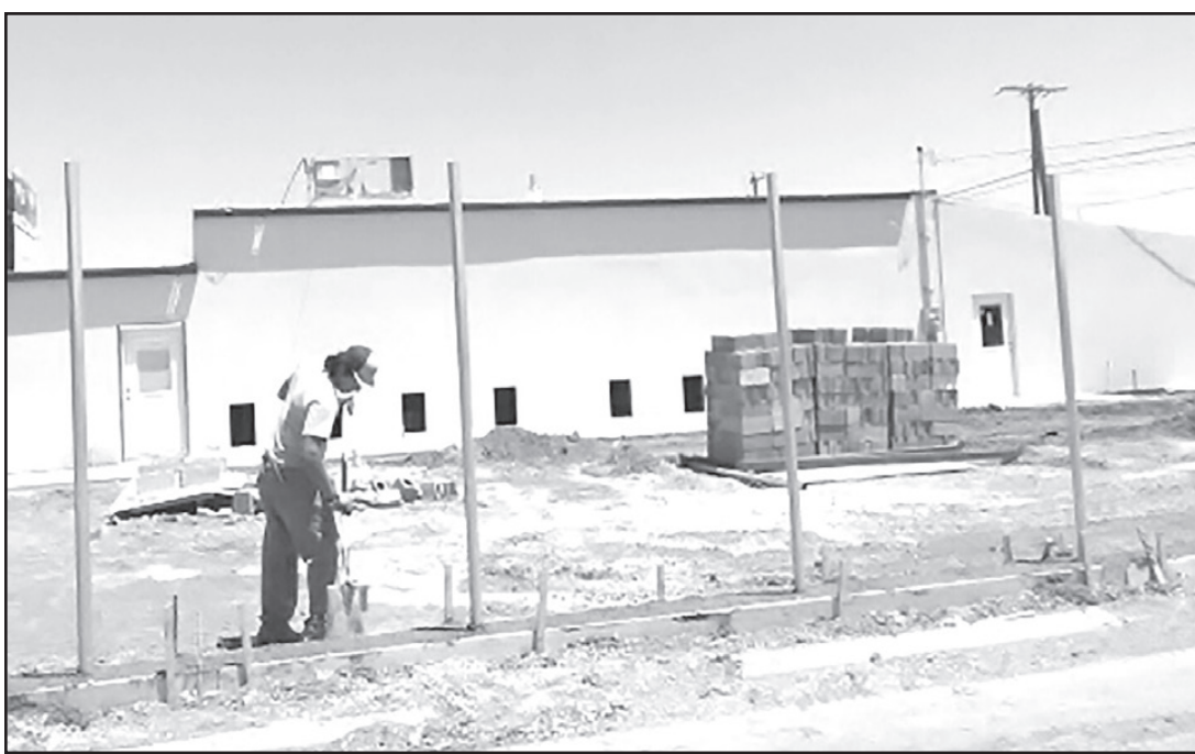
Work in progress on the back of Parmer Paws building—kennel openings visible
