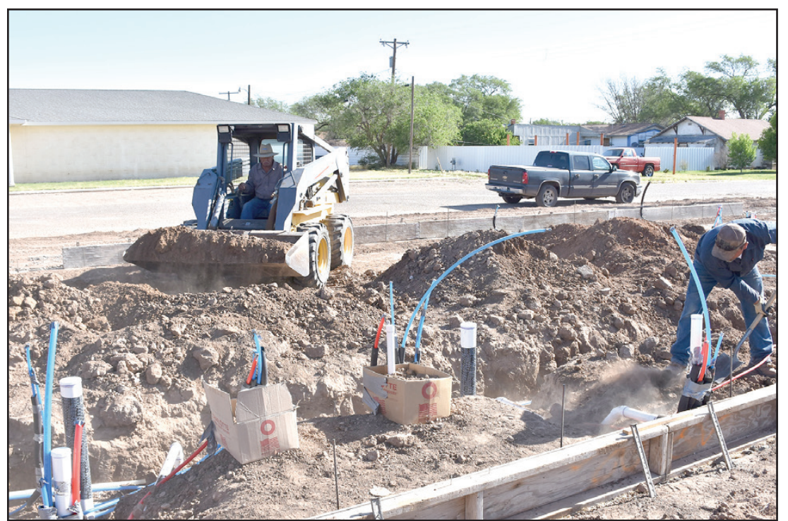
Construction work continues all around town. In the top photo, the original windows of the Friona Junior High have been removed and the openings boarded up until the new windows are ready to install. The middle photo shows work at the new Primary School site. The pad has been finished and the next step is concrete footings and grade beams. In the bottom photo, the plumbing has been installed and dirt is being moved to prepare for the installation of the slab.
