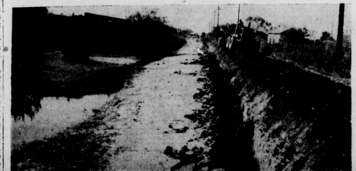
Pictured is one of the City's street and water department machines, used in street maintenance and as an all-purpose machine in back-filling water and sewer main ditches. Operator of the machine is Roy Oliphant, veteran employ in the street department.—(Photo by Blohm.)
