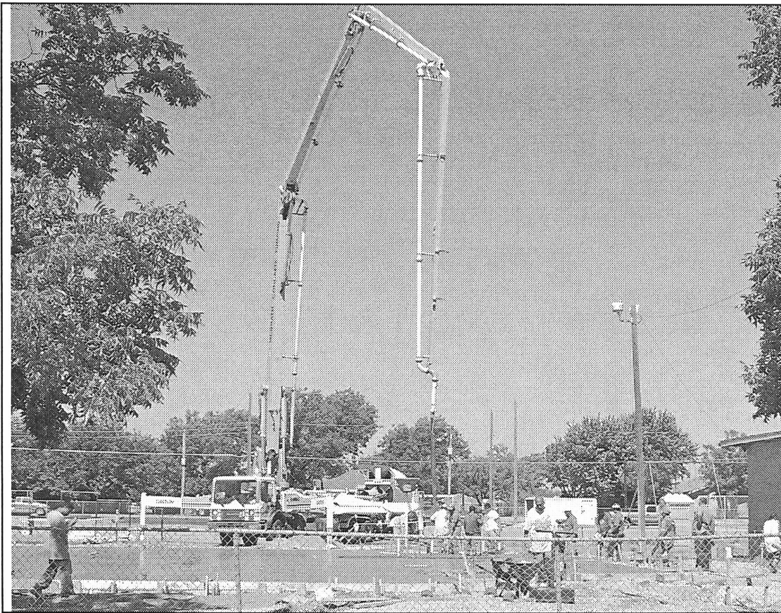
GYM START —Workers were scurrying to work the cement new multi-purpose facility being constructed at Haskell Elementary School.
