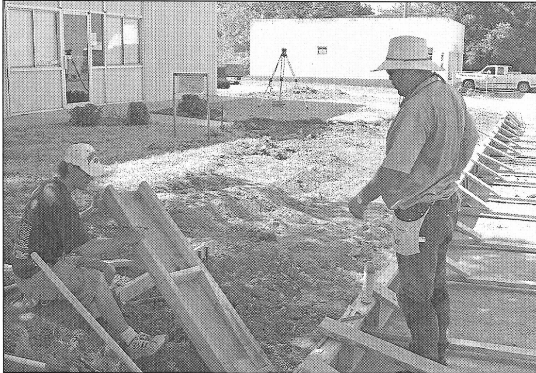
BETTER ACCESS —Dewayne Meier, left, and David Dodson construct concrete forms for the new sidewalk and approach in front of the Haskell County Extension Building
