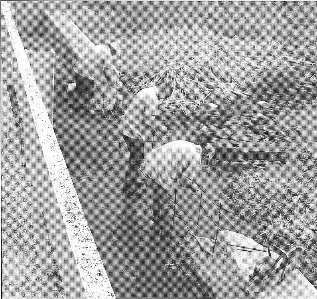
BEAUTIFICATION PROJECT —Haskell City workers are making forms to prepare for the pouring of concrete to repair the weir below the bridge along Avenue H. The weir holds the water allowing for ponding of the creek water making the creek's appearance more pleasing. Preparing the forms are, from top, Alfred Ozuna, John Wheat and Cory Green.
