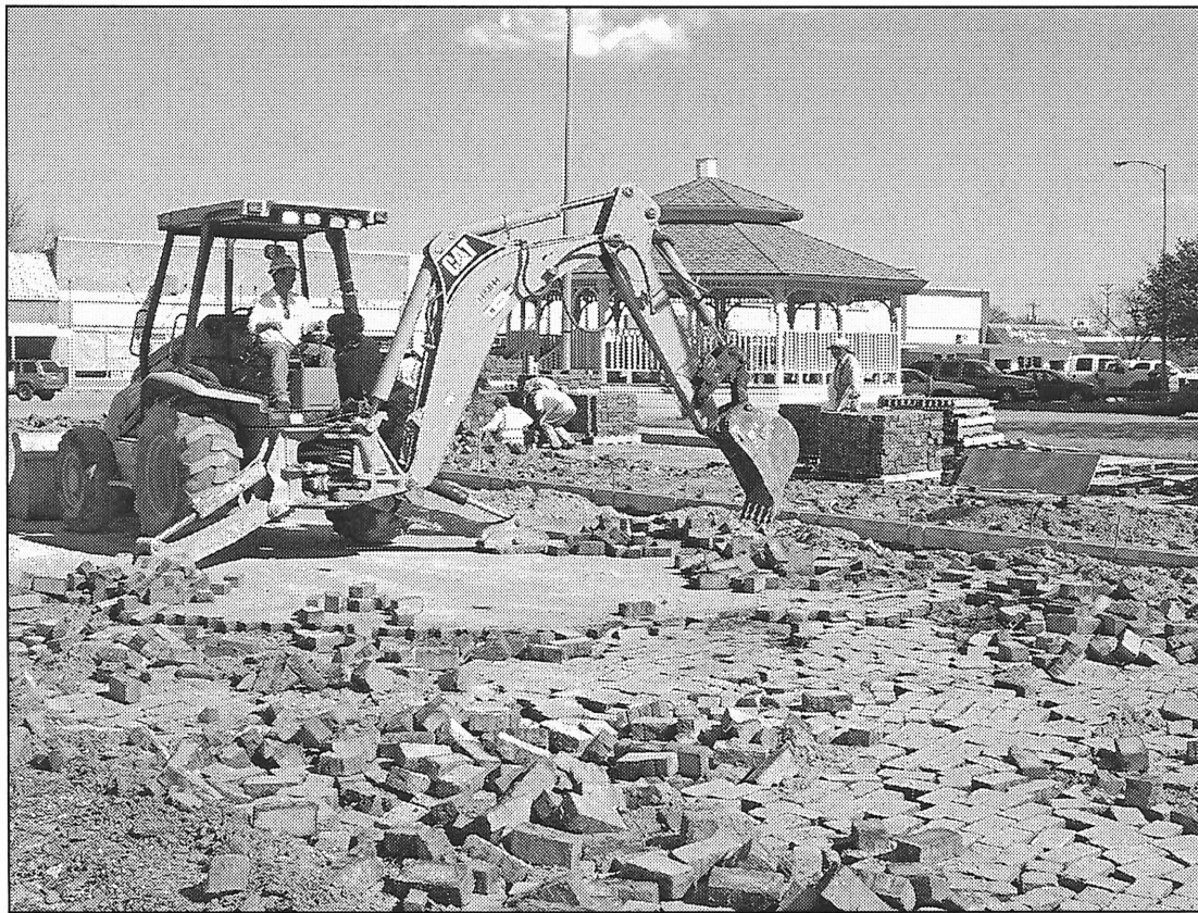
BRICK SALVAGE —Construction workers removed the bricks that have been hidden beneath the pavement around the square for many years for salvage. In the background workers palletize the bricks to save for relaying in the median area between the new curb and the courthouse sidewalk. Surplus bricks, if any, will be the property of Haskell County and may be used in decorative construction of the new Haskell County Library.
