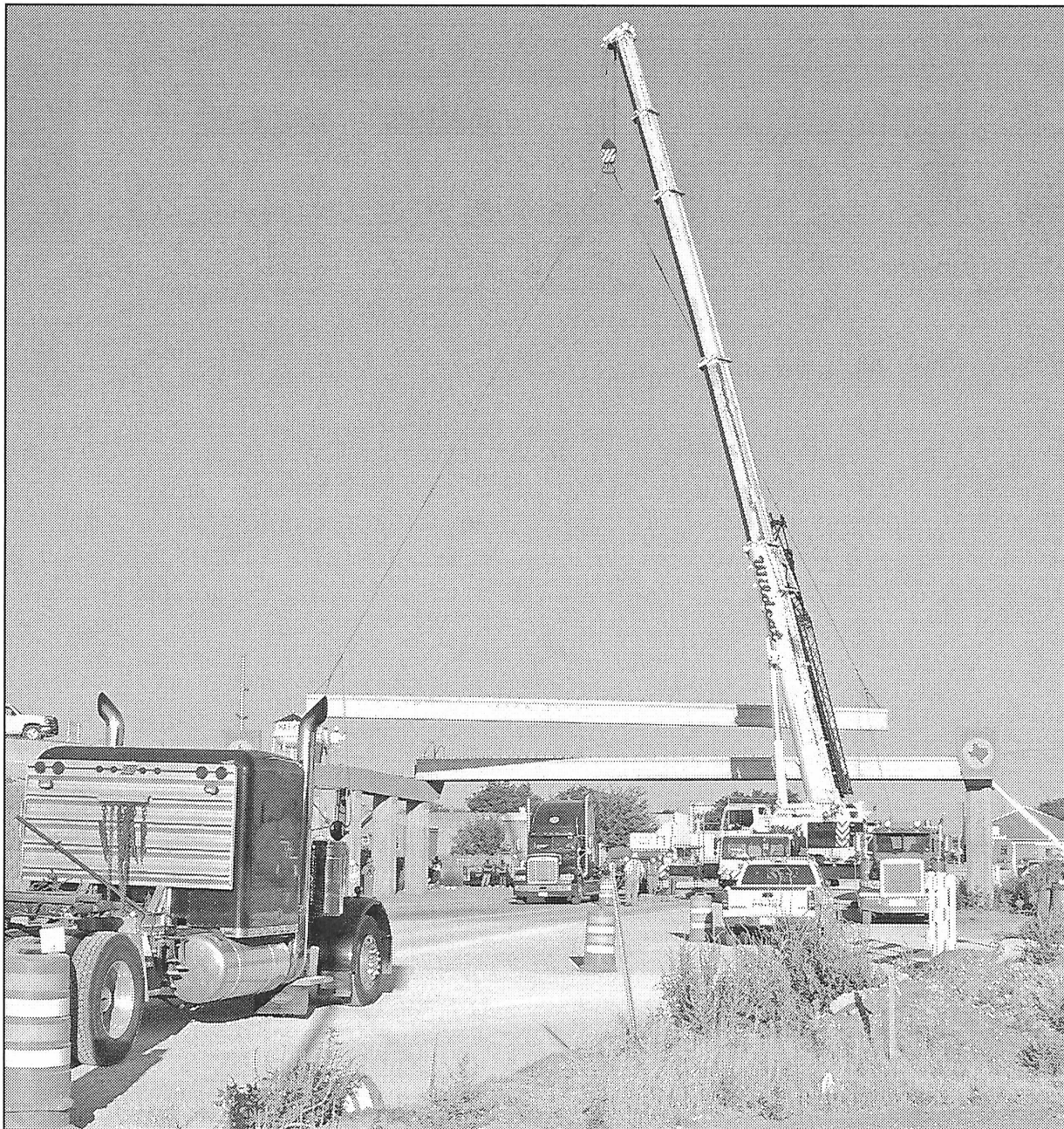
HASKELL'S NEW SKYLINE —Early Tues., July 25, Haskell's eastern skyline took on a new look. Construction crews placed 90' concrete beams across the roadway supports to join the two
