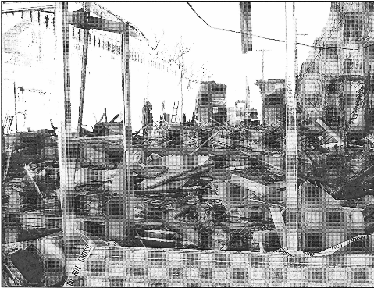
CLEAN UP AFTER THE FIRE —Work crews began the clean up of the Conner Floral building this week, located on the east side of the square in downtown Haskell. The building was determined
