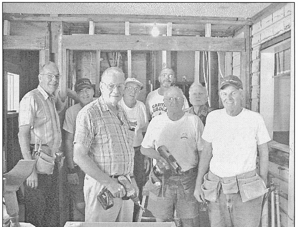
GOD'S OLD GEEZERS—Helping to repair a flood damaged residence at Veda's Camp last week were God's Old Geezers of First United Methodist Church in Garland. The men, front row l-r, are Harry Andreasen, George Jensen, Bill Bryant; back row, Dick Sutton, Dallas Windham, Max Benham, Scot Wingo and George Inman. The Haskell VOAD committee now has funds to make purchases of building supplies and hopes that more groups will be available to help with the repairs in the coming weeks.
