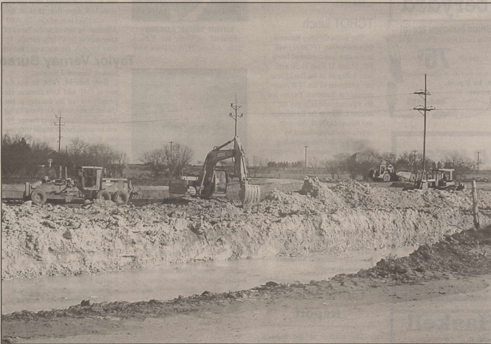
MAKING WAY FOR THE HIGHWAY —Construction crews and equipment were busy on South 6th Street in Haskell Monday, as it and several streets are closed, and work continues on the extensive Hwy. 277 bypass around Haskell.
