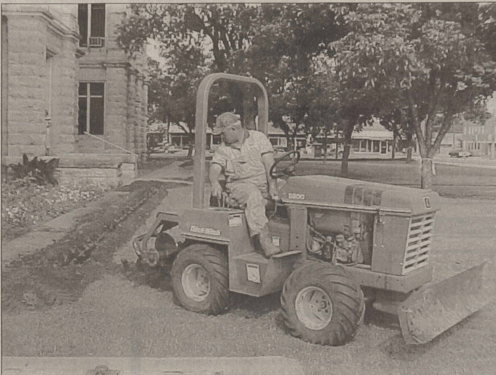
JUDGE 'DIGS' CHRISTMAS —Using a City of Haskell ditcher, Haskell County Judge David Davis works to dig a ditch for installing electrical lines for the extensive Christmas decorations that have been donated by the Allie Belle Smith family to be
