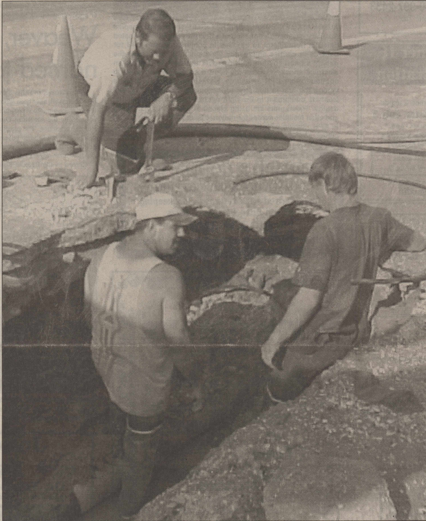
WATER WOES —Jerry Stanford, top, checks with Cory Green, left, and Kenny Bullard while they make repairs to the city water main on North 1st Street. Crews made repairs to five different water leaks during the late evening on Sunday and into the early hours of Monday morning. The city's main water tower is temporarily out of service with painting repairs. Use of one water tower is causing water pressure to fluctuate and aging water lines to burst keeping city crews busy. Relief valves are being used around town to help with the fluctuating water pressure.
