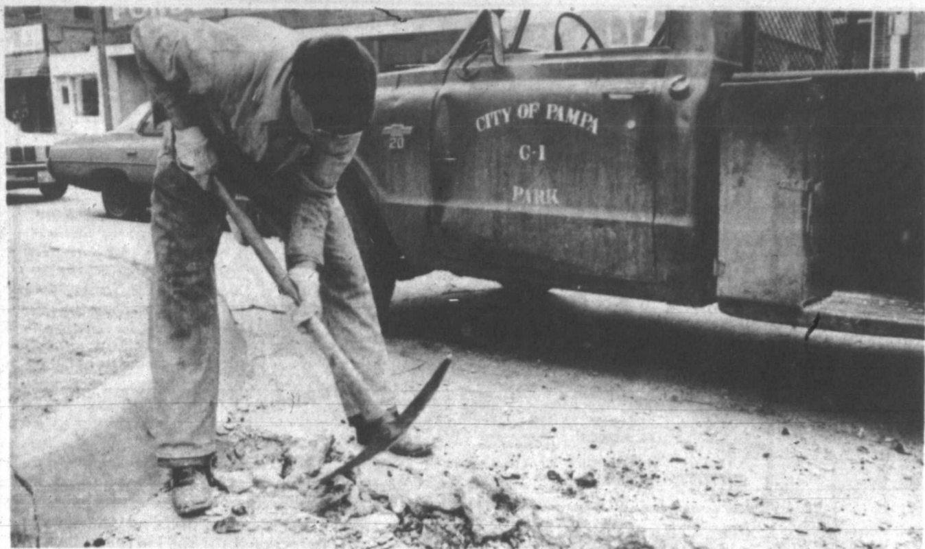
MUNICIPAL EMPLOYEES INSTALLED another two-inch water line at the city jail Wednesday afternoon to increase water pressure
