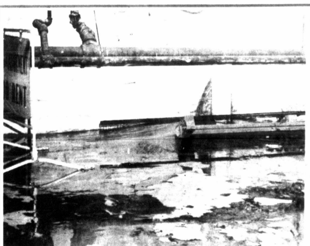
PAMPA HIGH SCHOOL auditorium often gets wet when there is heavy rain because of a leak. (Pampa News photo and story by Eugene Laycock)
