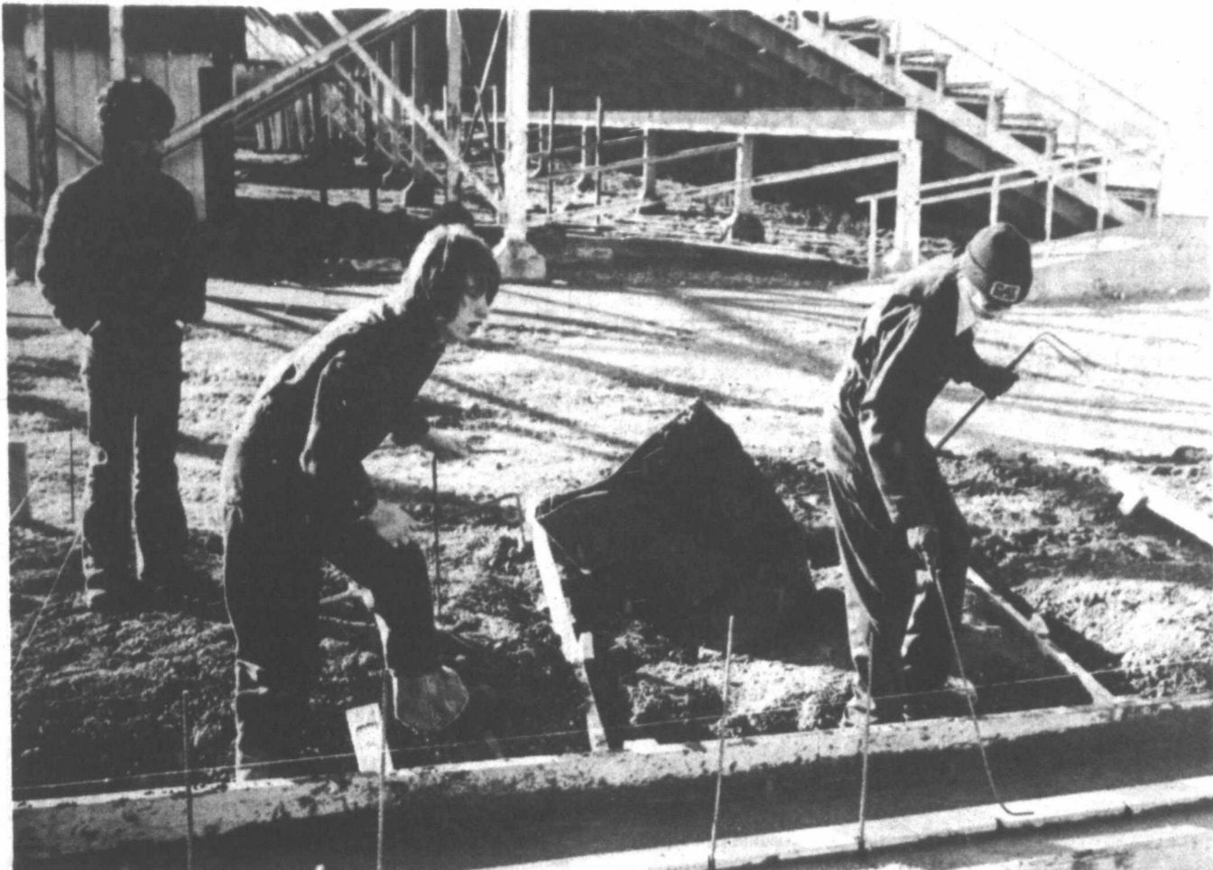
STUDENTS from Pampa High's Building Trade Class pour concrete for one of the new concession stands at the football stadium. (Pampa News Photo by John Price)
