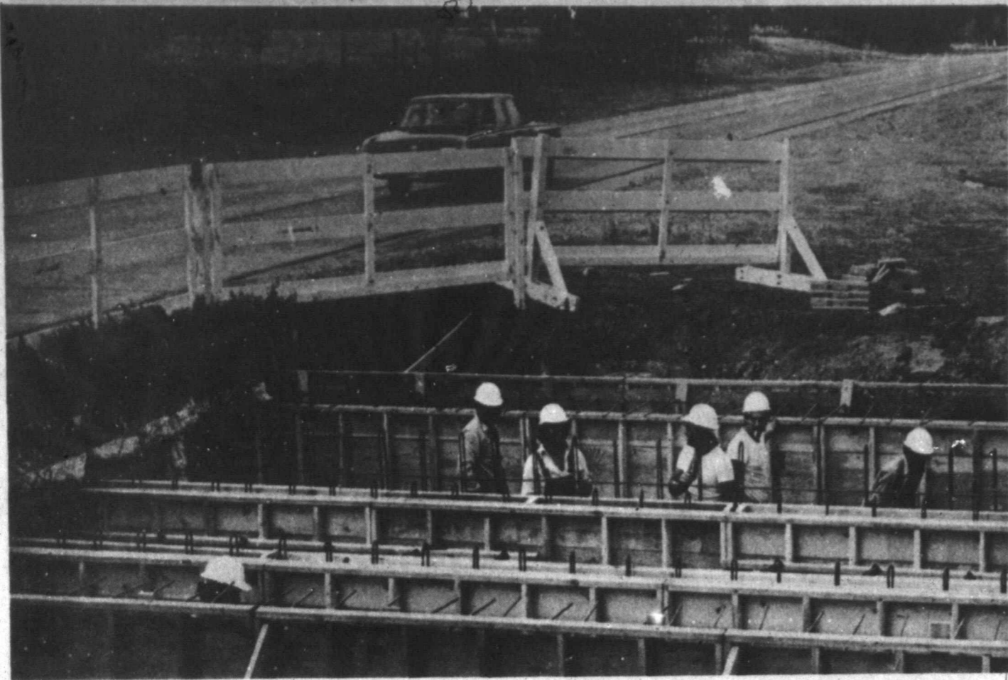
A CONSTRUCTION CREW from El Paso widens a culvert on Highway 83 north of Wheeler. The two-lane highway is being widened and resurfaced from
