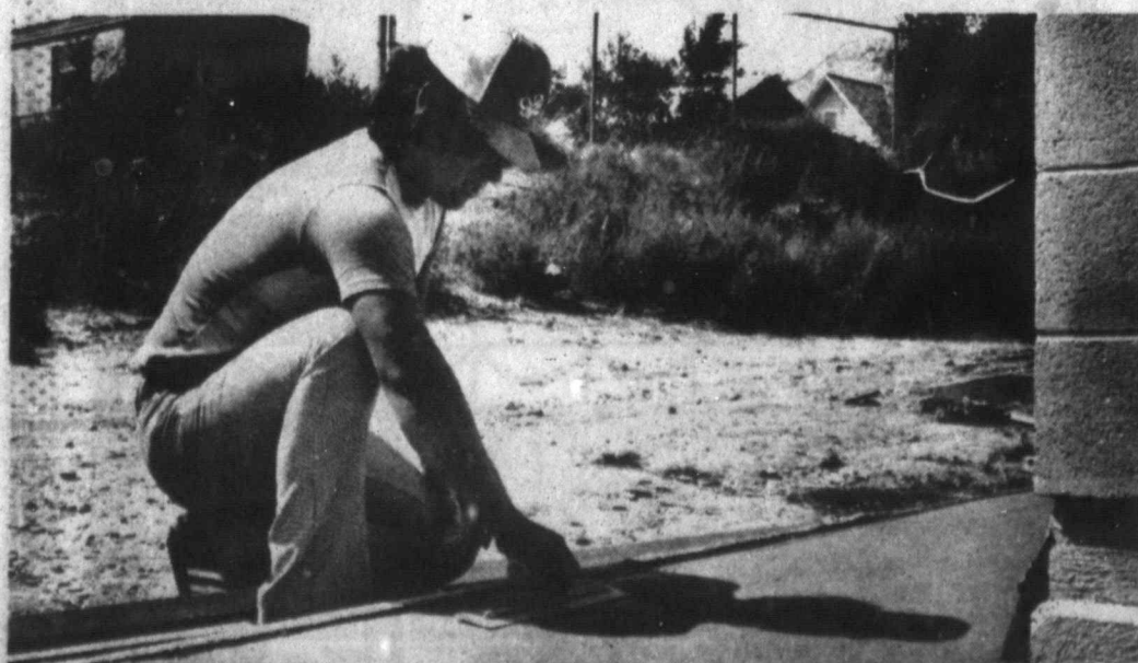
Pilo Sanchez smooths wet cement around the bath house at the new municipal swimming pool.
