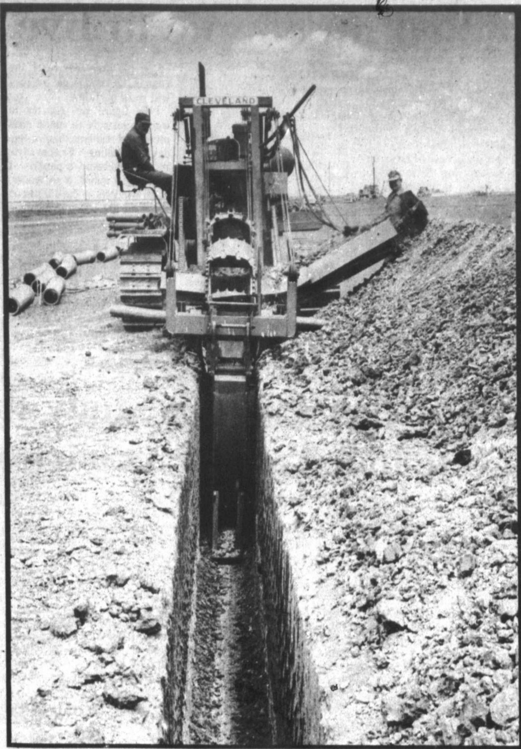
Digging is Progress Digging of sewage lines is still going on at the Pampa Mall site. All the underground lines must be completed before top construction can begin. (Pampa News photo by Ron Ennis)
