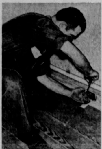
Sufficient convenience outlets are essential to comfort and safety.
