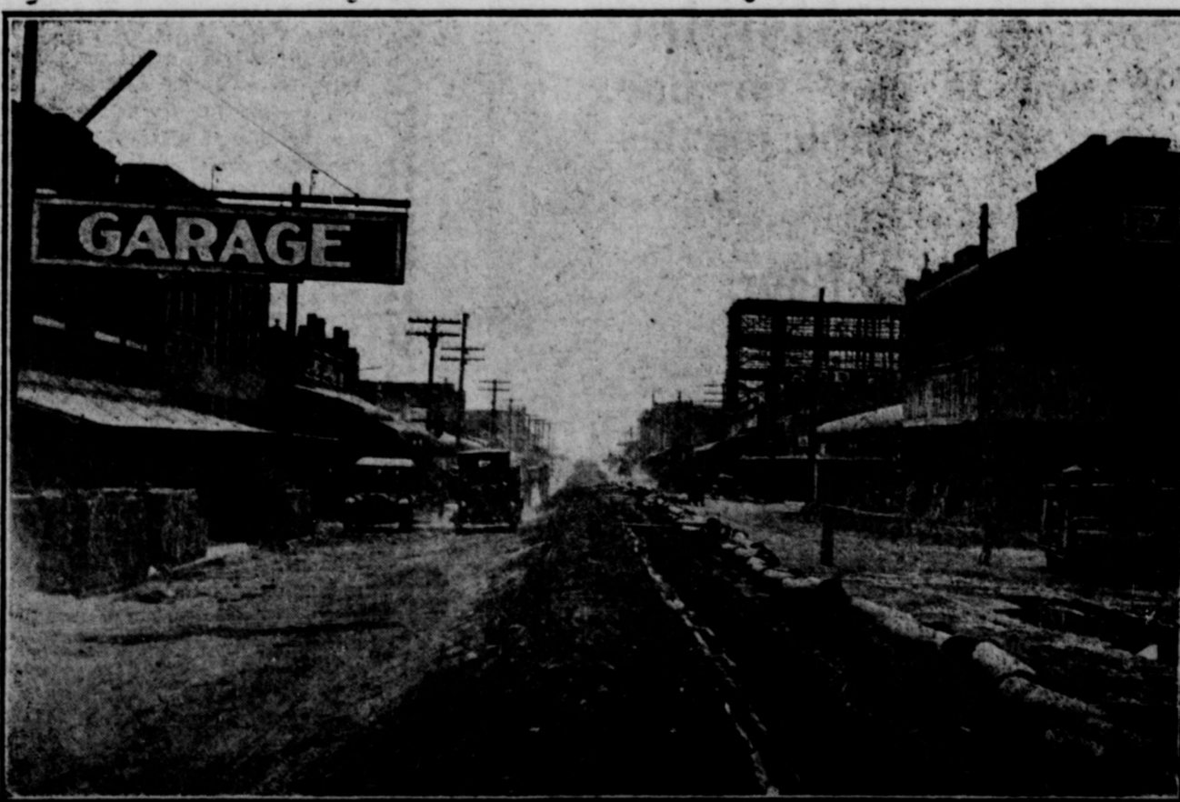
And as it looked three weeks ago, showing the excavation for the new 8 inch water main and many handsome business houses.
