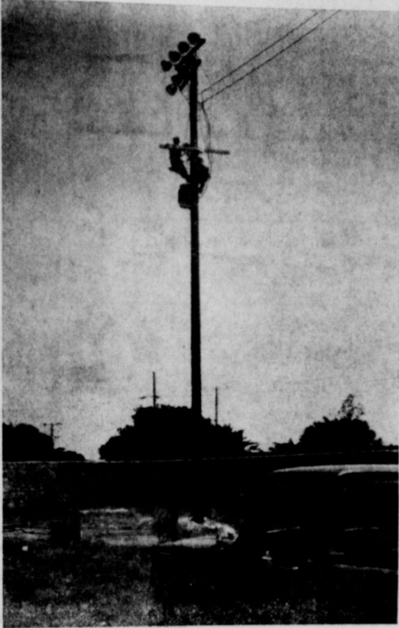
FINISHING TOUCHES — Community Public Service Co. linemen are shown putting the finishing touches on the new stadium lights, installed last week. The new facilities include ten new standards, each carrying eight fixtures. The old lighting system had only eight standards with 40 bulbs.
