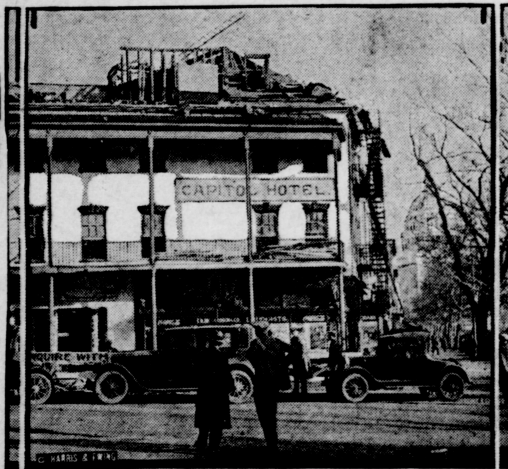
One of the real landmarks of Washington—the old Capitol hotel, on Pennsylvania avenue and within a stone's throw of the capitol—is being demolished to make room for a gasoline filling station. The sole surviving relic of slave market days in the national capital, an old auction block, is just north of the hotel.
