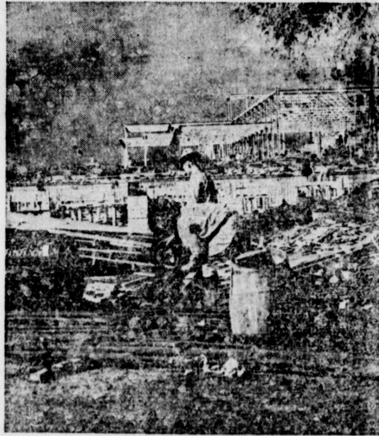
The steel frame of the $140,000 Livestock Building No. 2 for the Texas Centennial Exposition at Dallas can be seen above as it rapidly takes form. With the $260,000 Livestock Building No. 2, soon to be started, it will house the greatest exhibit of livestock in the nation's history when the Exposition opens June 6.
