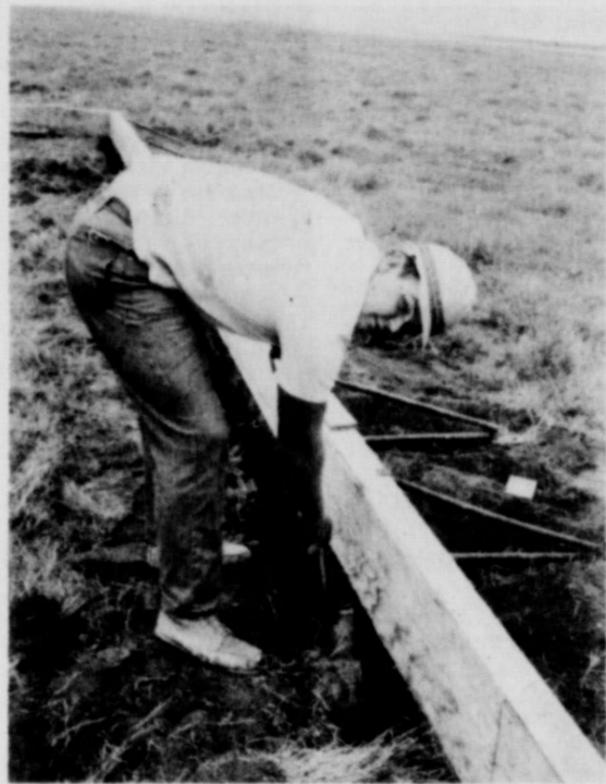
Ronnie Armstrong sets forms for the feed-mill foundation, at the new Hansford Feedyards in Spearman.
