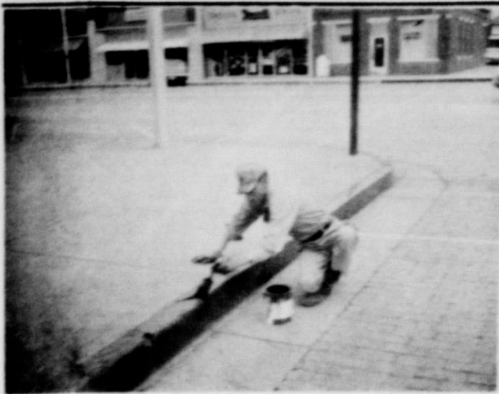
CLEAN-UP Campaign for the city has James Lantz, city employee, putting a new coat of paint on the parking areas in town. The work began Wednesday.
