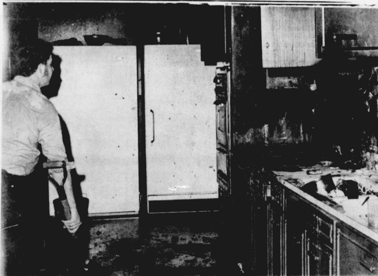
SURVEYING THE DAMAGE-- An unidentified fireman surveys the damage caused in the kitchen of the Gordon Crouch residence in a rural area of Hockley county. Morton Volunteer Firemen
