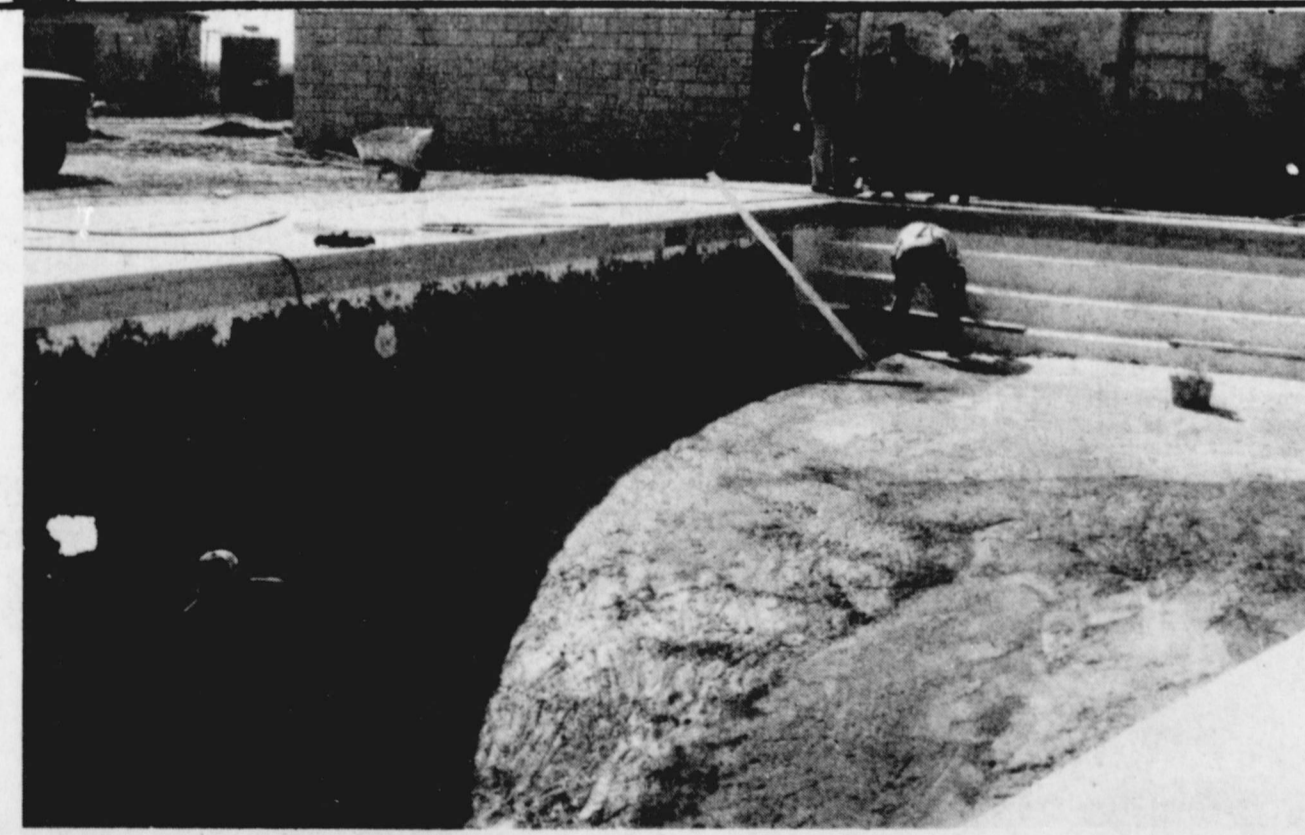
WORK WAS PROGRESSING rapidly on both the swimming pool and the club house addition at the Morton County Club when this photo was snapped several days ago. The pool has since been completed
