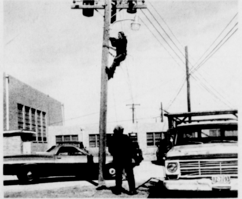
THE CABLES ARE COMING, gerump, gerump. Workers are shown in the alley behind the county activities building Monday as they began laying the wire for cable television which is expected to become operational by April 15. The cable will serve all the homes in Morton and provide closed circuit broadcasting facilities for the Morton schools and the county activities building.
