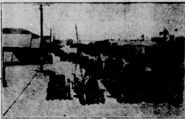
Trucks of L. P. Yocham hauling line of pipe to the Yates Pool.
