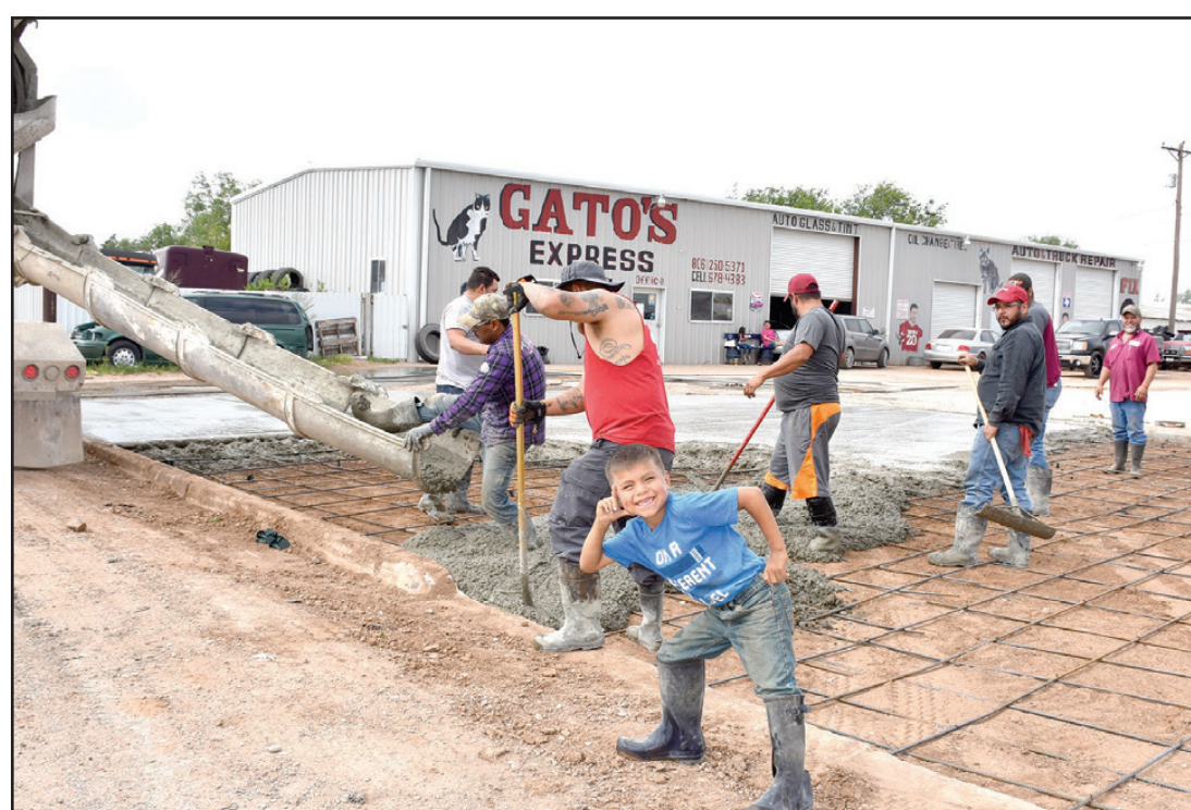
Uriah Monreal is shown "directing" the work crew pouring new concrete at Gato's Express. Antonia Monreal is the owner and has been in business for approximately ten years.
