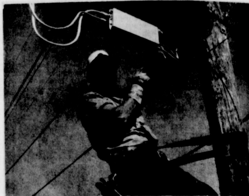
Scenes such as this have become a familiar sight as construction nears completion. R. D. Treloar makes a final signal adjustment.
