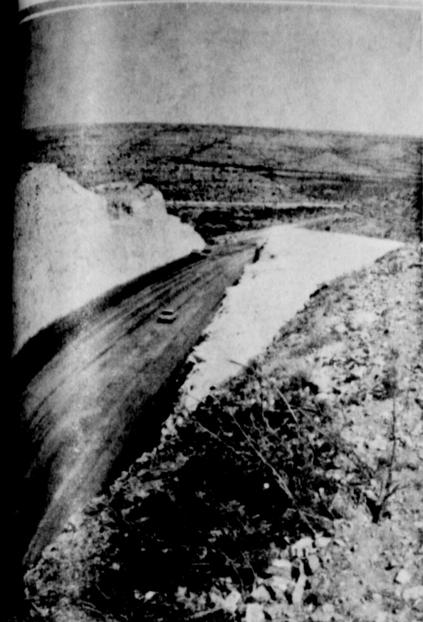
Pictured above is a view of the new roadbed from the top of "Big Hill" looking north. The cut is 35 feet deeper than the old road which can be seen as the white patch on the right and the cut on the left and winding from left to right in the distance. Crews moved over 2,500 cubic yards of dirt daily from the cut scheduled for completion before October 1, according to Kenneth Plunkett, resident engineer on the project.
