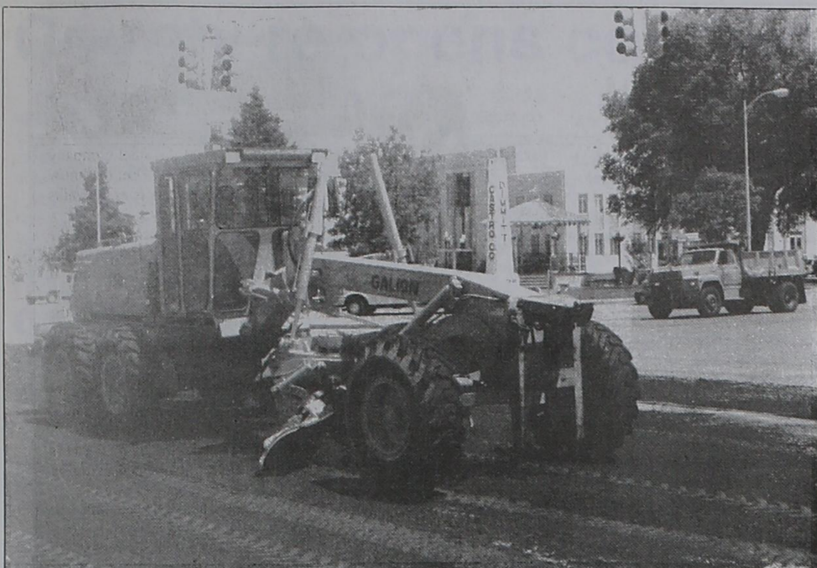
MAJOR INTERSECTION GETS SMOOTHED OUT —Workers with the Texas Dept. Of Transportation closed the intersection of US Highway 385 and State Highway 86 on June 7 to smooth out the intersection. The top of the roadway had been bladed
