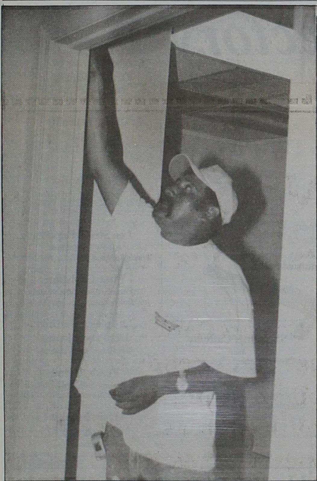
CONSTRUCTION AT THE NEW CLINIC—Louis Alvarez puts the finishing touches on paint around an interior door frame at the new offices for the Medical Center of Dimmitt, located in the 100 block of West Jones in Dimmitt. When complete, the offices will house three physicians, two mid-level practitioners and support staff. Photo by Anne Ackers
