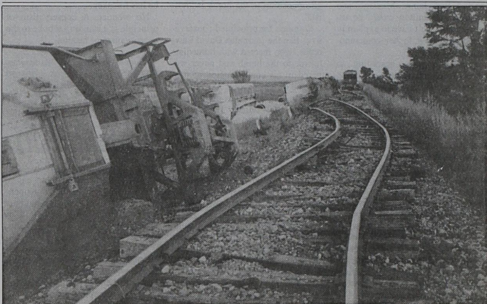
HOPPING HOPPERS —Eight cars of a Burlington Northern train derailed east of Hart around 5 p.m. Tuesday, damaging an estimated 800 feet of track. Some of the corn carried in the cars was spilled, but there were no injuries. The track was expected to
