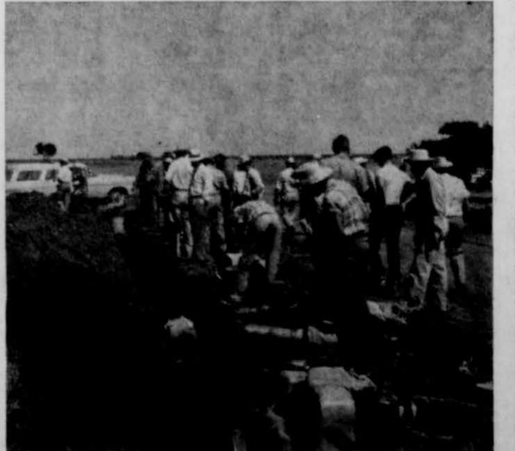
125 people were present for the dinner at Frio. Right, the farmers on tour inspect installation activities of a Brown Supply Company crew putting in the necessary equipment for irrigating out of a surface lake on Jay Boston's farm in the Frio community.
