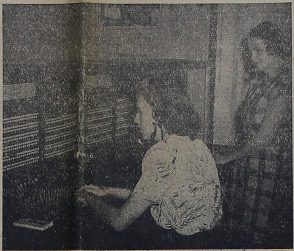
Pictured above at the new large switchboard, at the West Texas Telephone Company office, are Miss Jean Thomas, seated, and Mrs. Homer Hyatt, Chief Operator.
