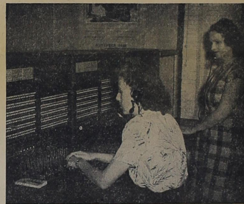
Pictured above at the new large switchboard, at the West Texas Telephone Company office, are Miss Jean Thomas, seated, and Mrs. Homer Hyatt, Chief Operator.
